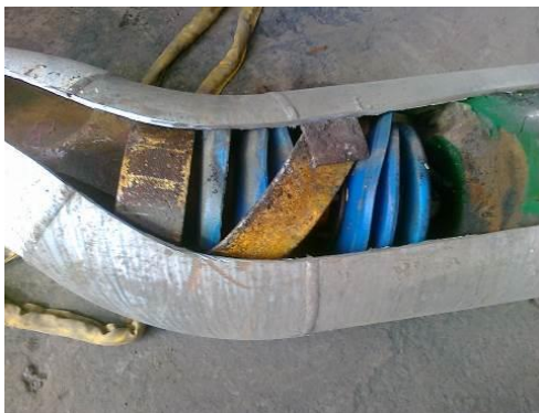
Cleaning Pig Stuck In Bend
