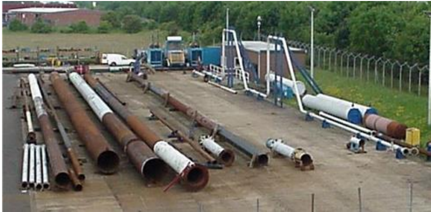
Figure F4.1 Pull through pipe spools with machined defects
